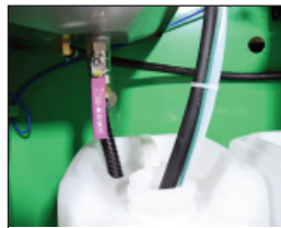
Drain Valve - Open
